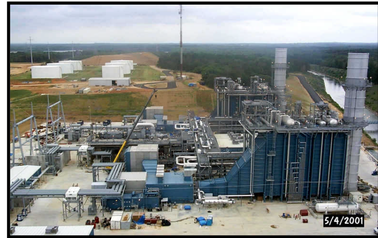
Gas Turbine Combined Cycle Plant
